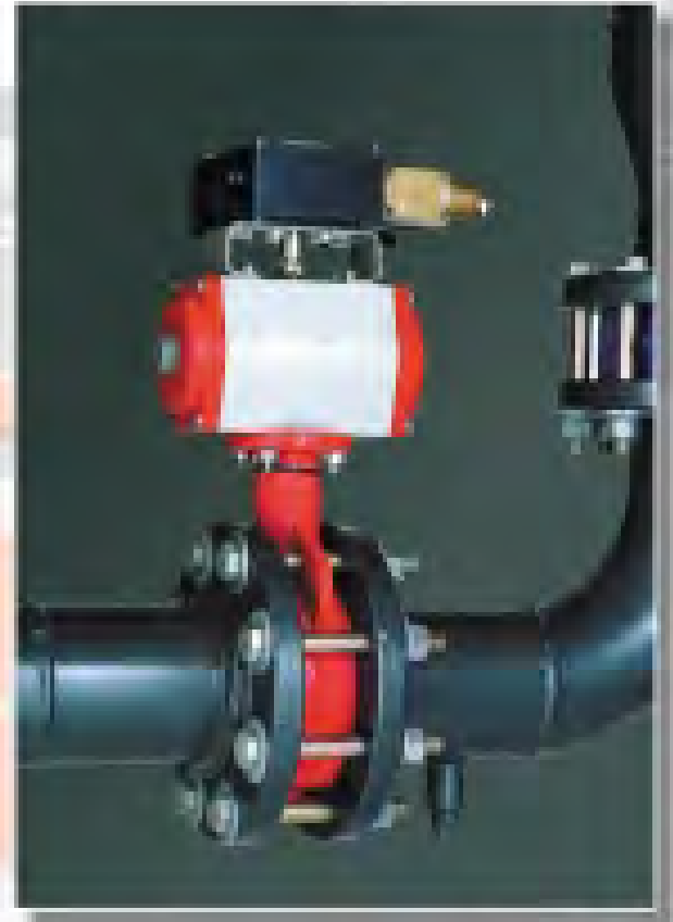
Flow Control Valve and Positioner with Actuator
